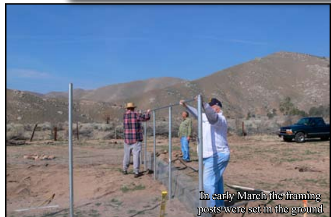
Reed, Bill, Bob, and Darrell trenched the water and electricity to the enclosure in November
